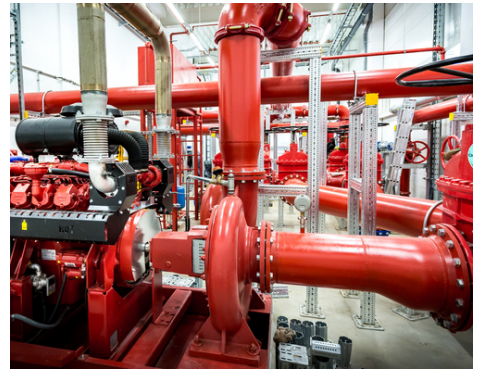
Fire Protection Systems
