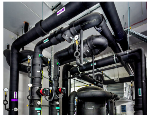
Heating & Cooling Installations
